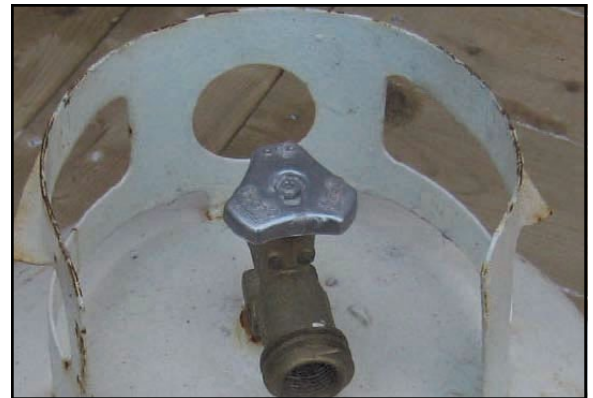
Only propane tanks with a triangular-shaped control handle have an excess flow valve .
